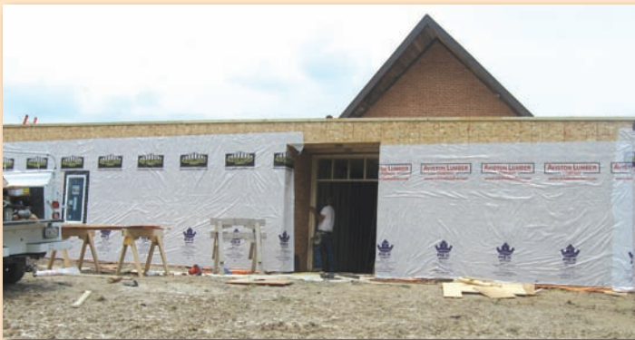
An addition of 1,500 square foot of space was added for the growing facility.
